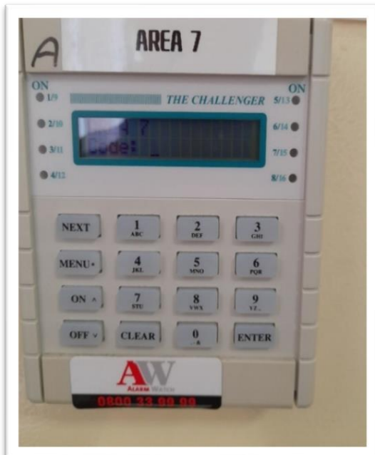
Image 2: Location of the Alarm keypad is at the entrance of the English Block/ Breeze way
